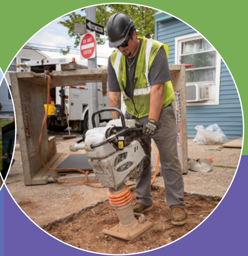
Mark Kehlenbach, a Utility Tech in our Construction & Mains Department, at a job site in New Haven tamping a water line trench.
