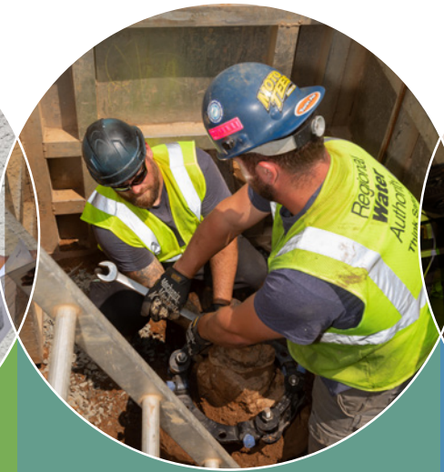
Our Water Mains & Service and Construction crews perform a lot of complex work every day on our more than 1,700 miles of pipeline to improve water service reliability. Anthony Spero (left) and Anthony Dellacamera , both Construction Utility Techs , work on a gate valve in North Haven. Projects like this avoid service disruptions and reduce water waste caused by leaks.
