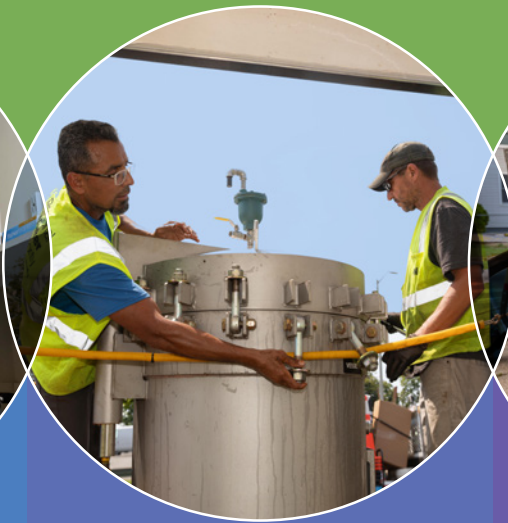
Ramon Cruz (left) and John Waligroski, both Utility Techs from our Construction & Distribution Department, preparing our new closed-loop water main cleaning equipment called NO-DES, an innovative method of cleaning mains with insignificant water loss, making it environmentally friendly.
