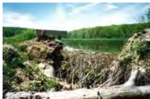
Beaver Dam in Spillway
