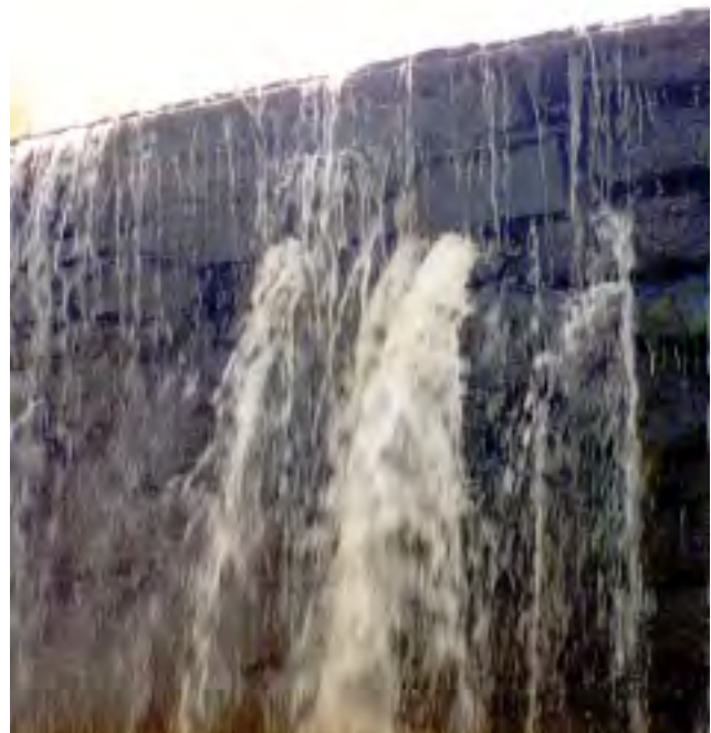
Leak in Masonry Wall
